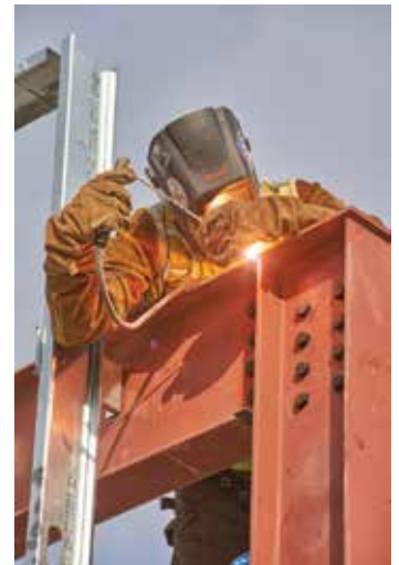
Connector John Carroll welds a moment connection at the Wellwood Middle School addition in Fayetteville.
