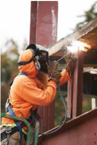
Connector Travis Richardson, a Marine Corps veteran, installs bar joist reinforcements at the Fremont Elementary School addition in East Syracuse.
