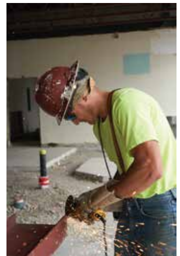
Crew leader and former Marine Eric Drewel end-preps a beam at the Fremont Elementary School addition in East Syracuse.
