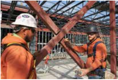
Pictured from left are crew leader Mike Perez and connector Jim Ormsby inspecting a tube brace at the Wellwood Middle School addition in Fayetteville.
