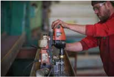
Welder/fabricator Nick Kenney installs holes in channel members for the renovation of the Binghamton Armory.
